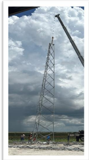
Hill County Communications Tower in Penelope built with State Radio Infrastructure Grant Funds
